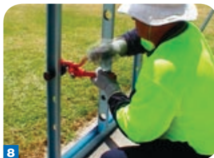
8 Or use the pre-made service holes already provided in the frame studs as pilot holes for the large punch.
