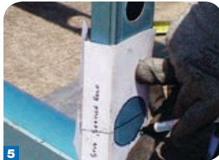
5 When cutting a penetration hole in a boxed stud, use a pre-made template to position a hole at your measured line on either side of the stud. Mark the holes on both sides.
