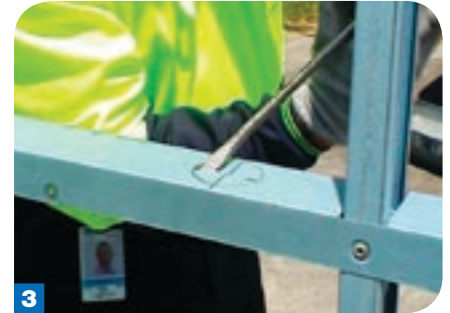
3 Use a screwdriver to open an entry point for the snips, and then, cut out with either your left-cut or right-cut snips.
