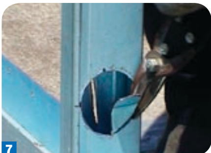
7 Finally, use your left and right snips to cut out the circles from the top down.
